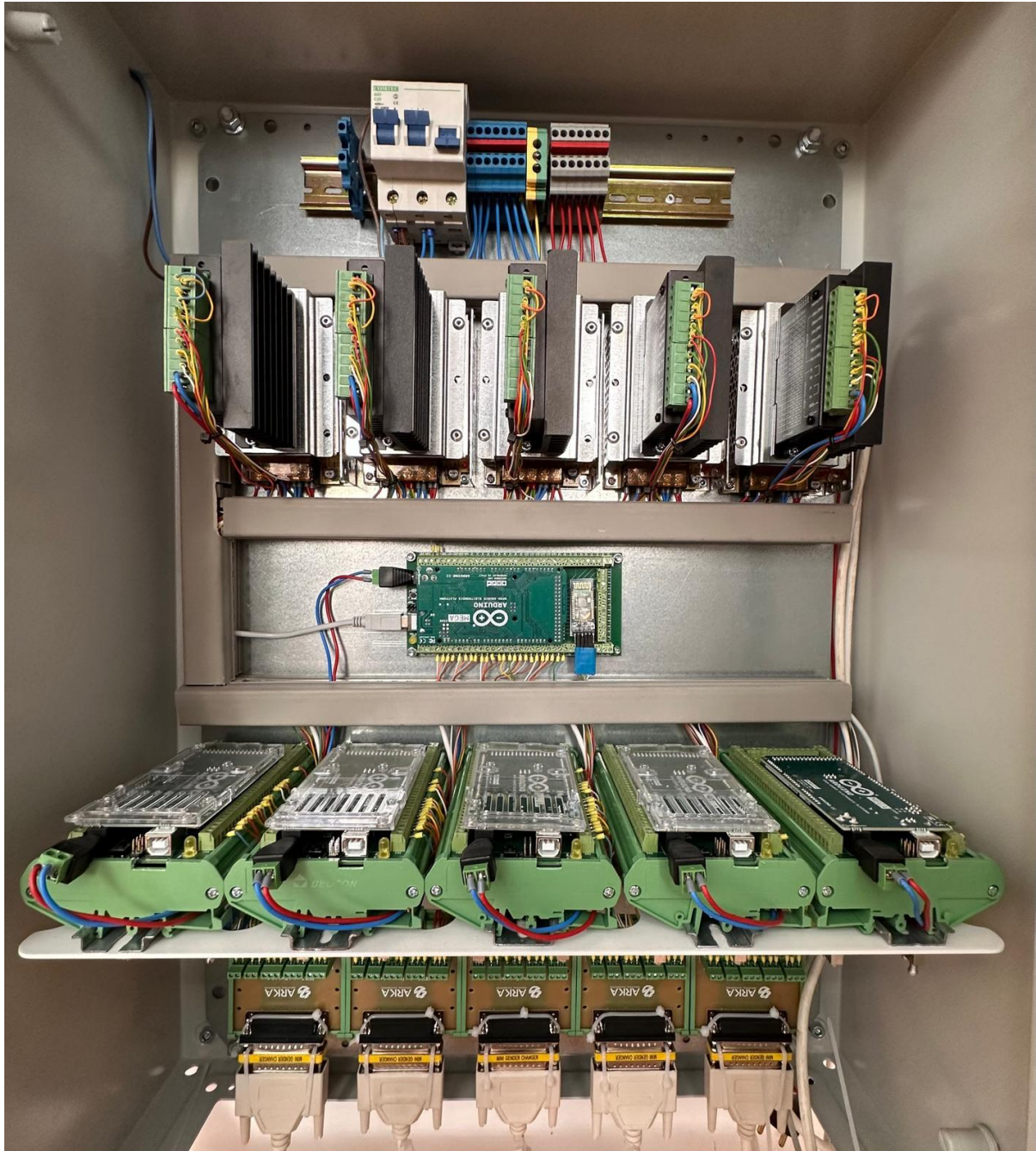
Figure. 5.17. Physical realization of the electrical panel
