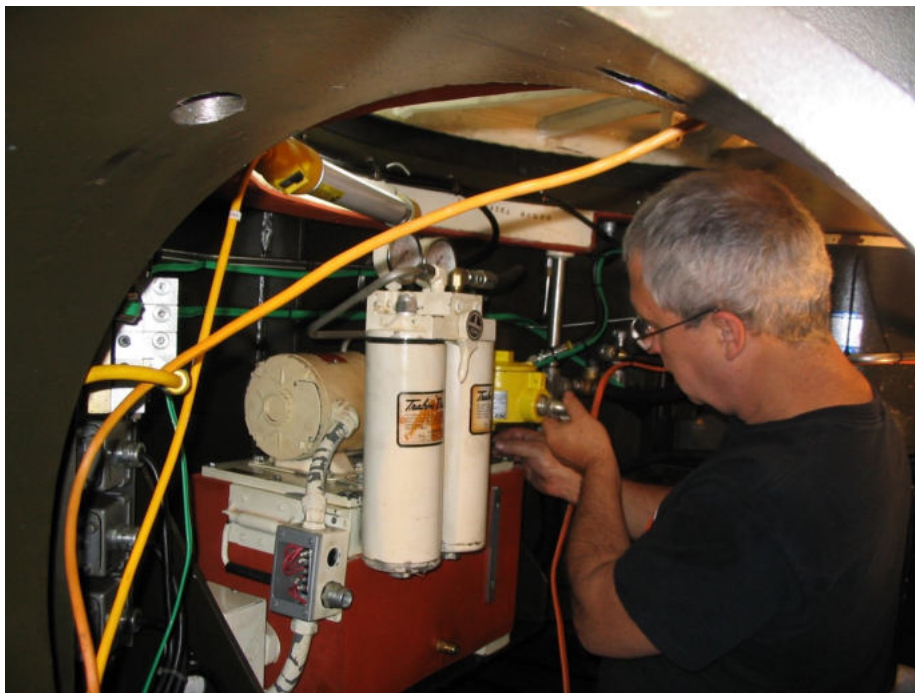
Figure 6.1 Technical area of the rotating system visually inspected by the technician
