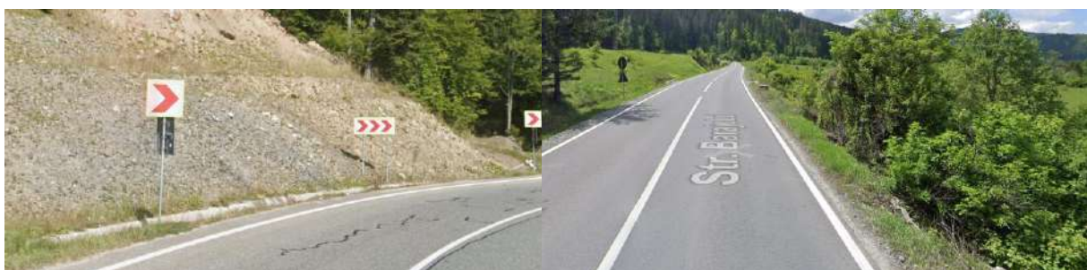
Fig. 2.7 Examples of hazardous cut and slopes
