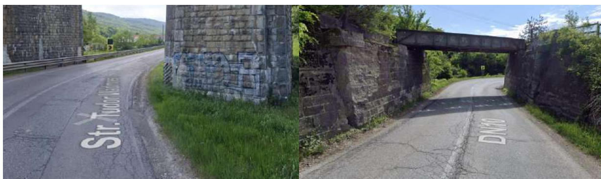
Fig. 2.3 Examples of hazardous bridge abutment and walls
