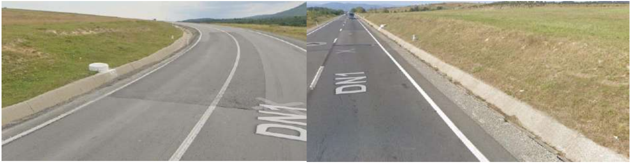
Fig. 2.8 Examples of hazardous roadside ditches
