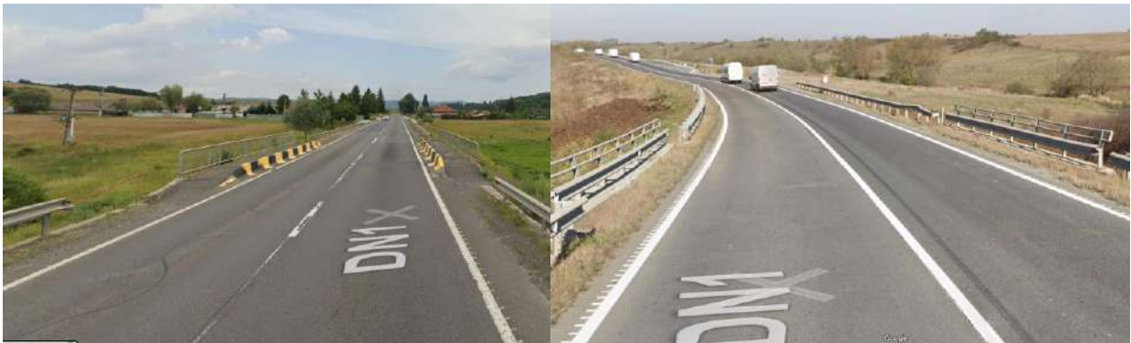
Fig. 2.4 Examples of hazardous safety barriers ends
